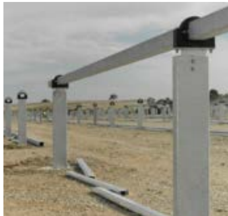
Image 34: Spherical bearings installed in Zuera 11 MW, Zaragoza
